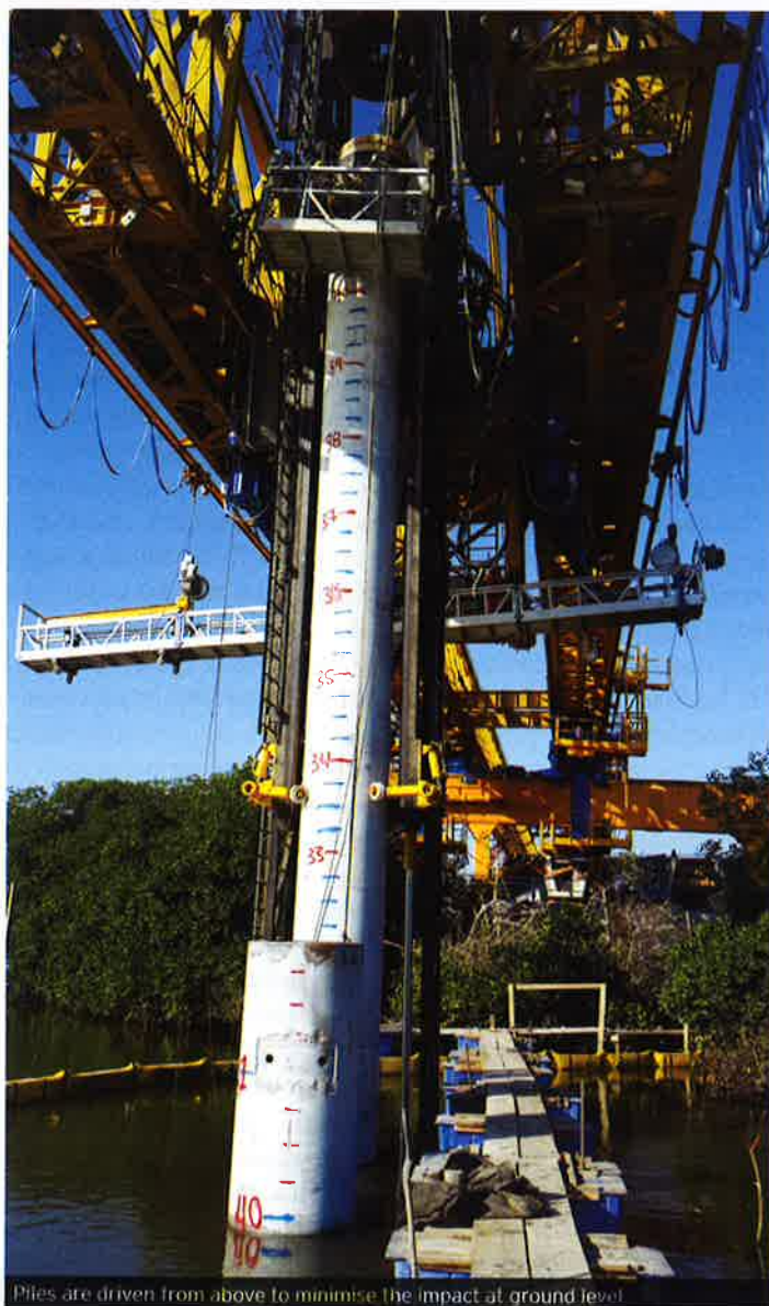
Piles are driven from above to minimise the impact at ground level
