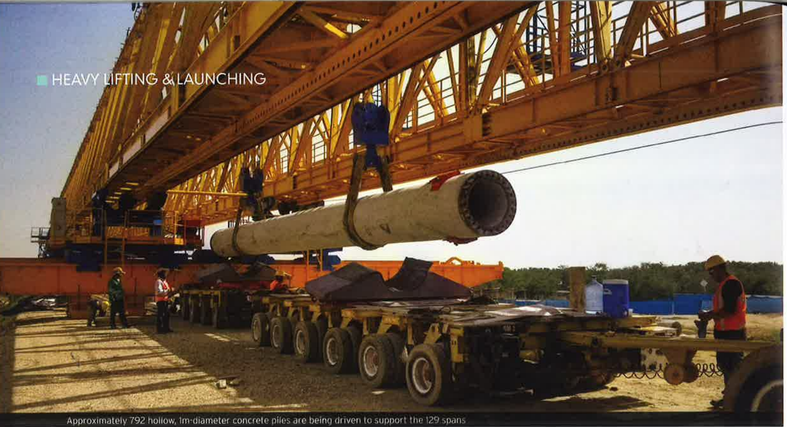
Approximately 792 hollow, 1m-diameter concrete piles are being driven to support the 129 spans
